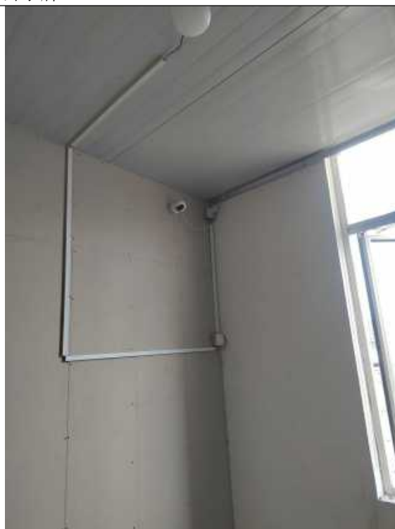
危废仓库防爆灯和摄像头
